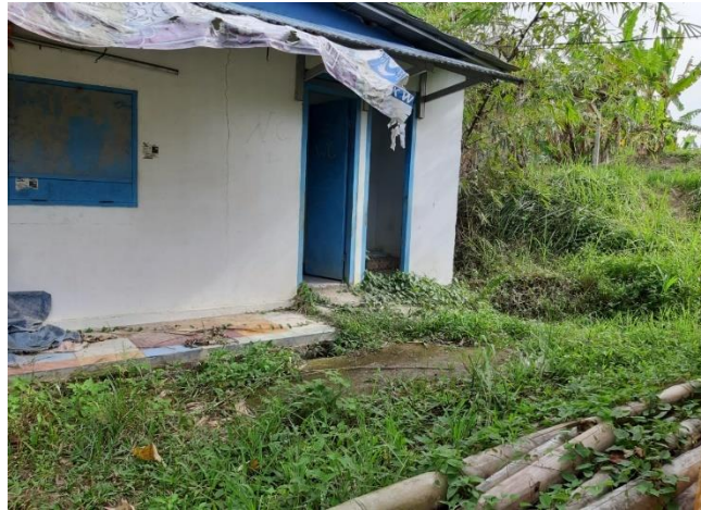
Gambar 4. Keadaan Toilet Telaga Biru Cisoka
